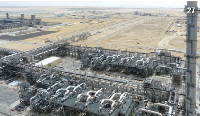
27. Manifa Gas Facilities Project 위치: Khursaniyah, Saudi Arabia - Gas Inlet Facilities, Gas Processing: 90 MMSCFD - Condensate Stripping: 66,400 BPSD - SRU: 900 TPD×2 공사기간: 2008. 08 ~ 2011. 10
